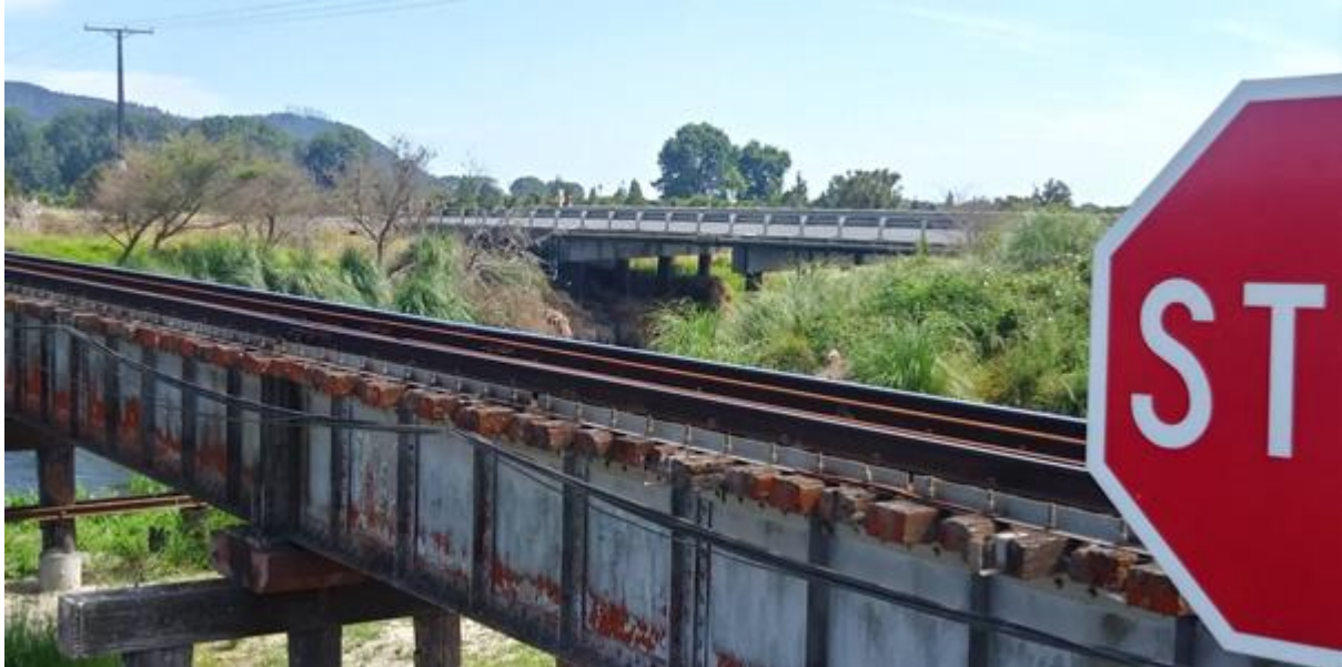
Fig. 12. (top) State Highway 2 Road Crossing and (bottom) Rail Crossing, with co-located network cables, at Tarawera River.
